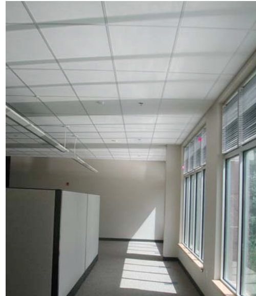
Figure 3: Daylight redirected by LightLouver units onto the ceiling
